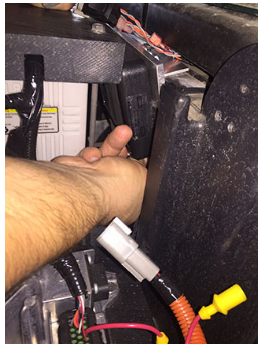
Fig. 21 – Wires leading from batteries
