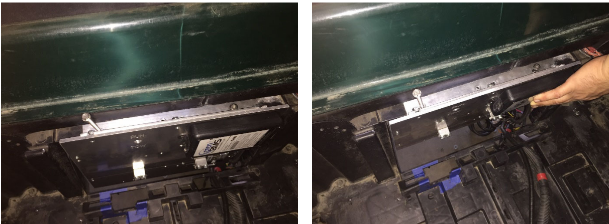
Fig. 17 – Fully assembled controller plate installed
