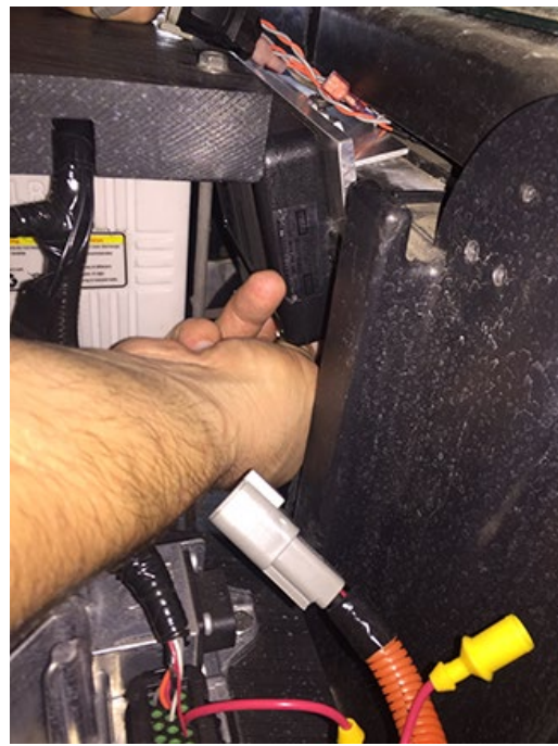
Fig. 21 – Wires leading from batteries
