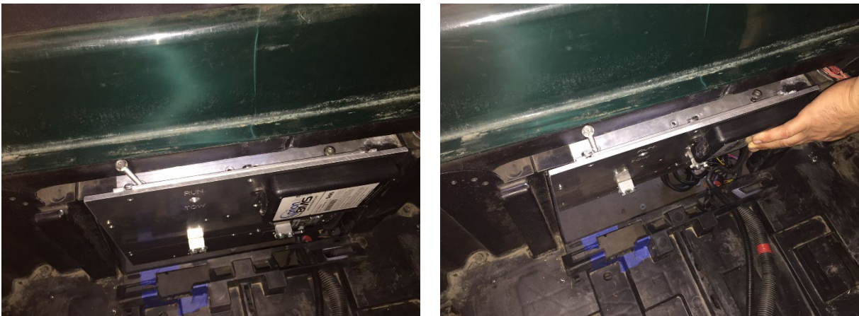
Fig. 17 – Fully assembled controller plate installed
