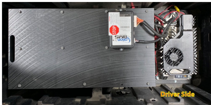
Fig. 1-Lithium battery pack installed into golf car
